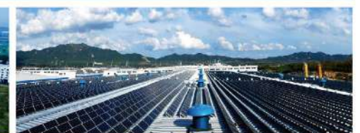
Solar panels arrays
